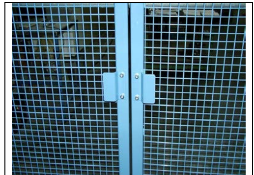
Opening landing level swing doors
